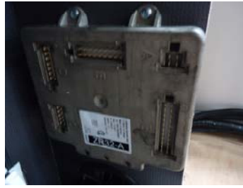
1. Central control electric box
